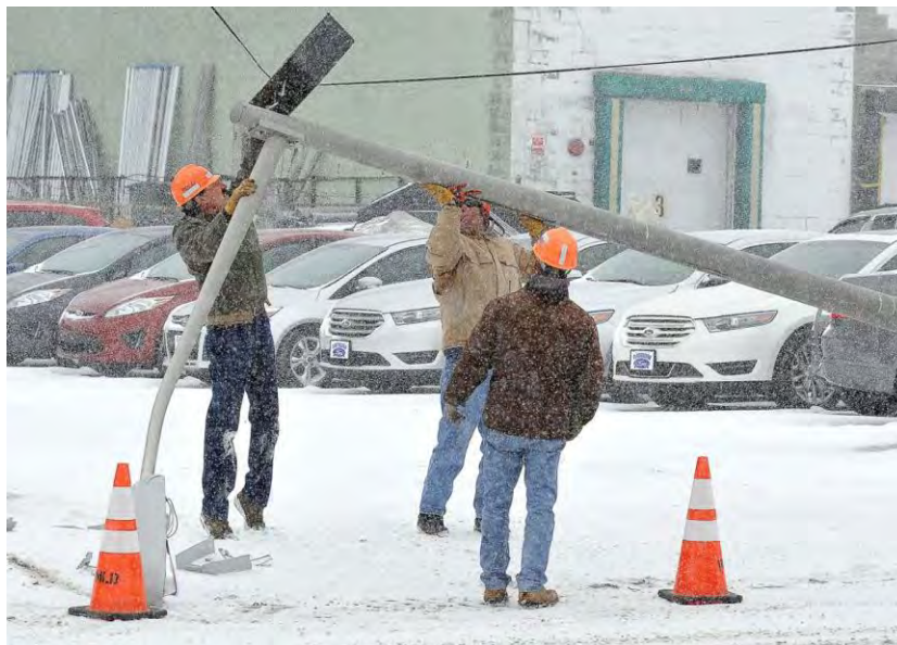
Winter driving conditions often cause cars to slide off the road. Plattsburgh Municipal Lighting Department personnel removing a struck light pole in the middle of a snow event in March 2014. (Press Republican)
