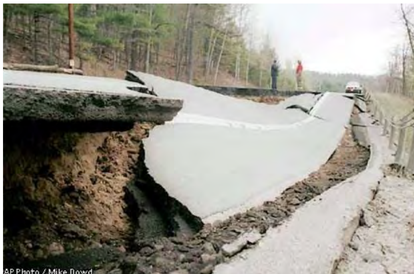
Images shows a section of Route 9N that collapsed 12 miles south of Plattsburgh as a result of the 2002 earthquake.
