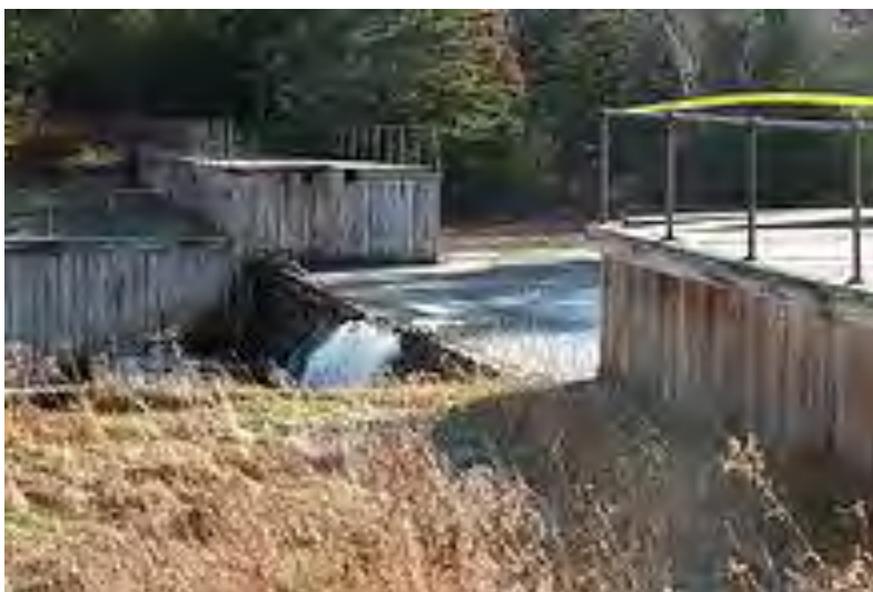
Marcy dam after Tropical Storm Irene
